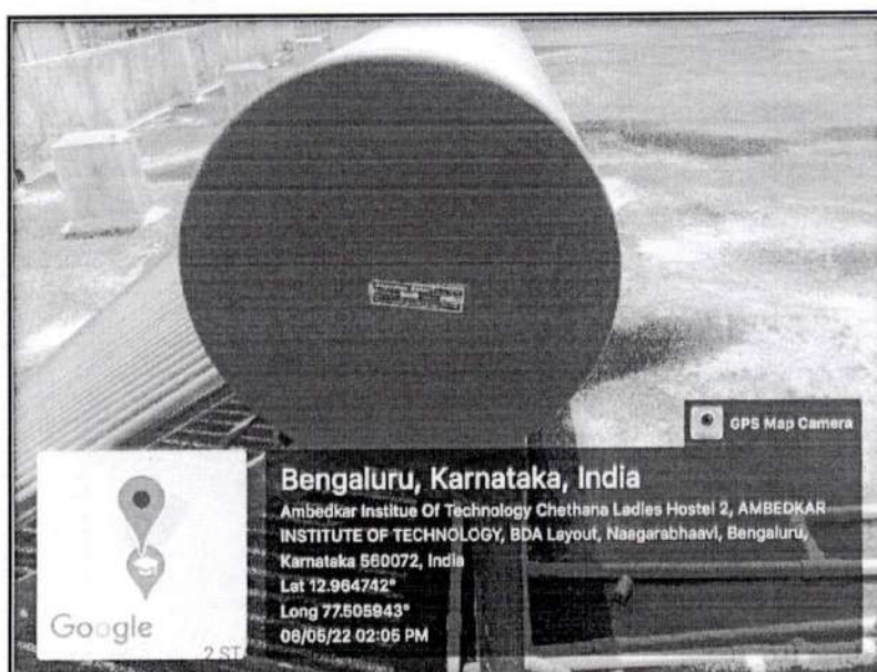
Photograph of Solar Thermal Water Heating System:
